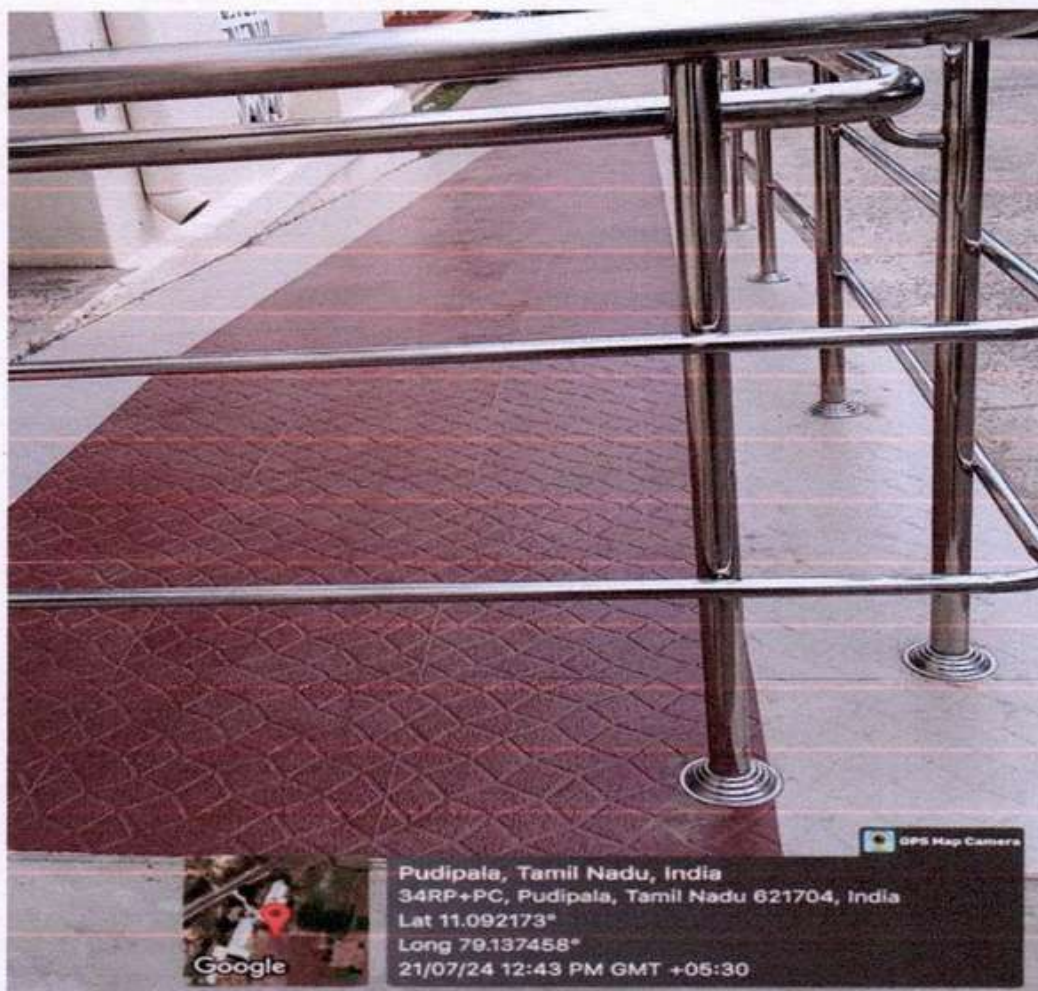
Ramp for physically challenged people
